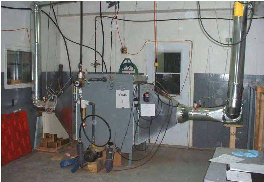
Figure 3. A picture of the air cleaning system.
